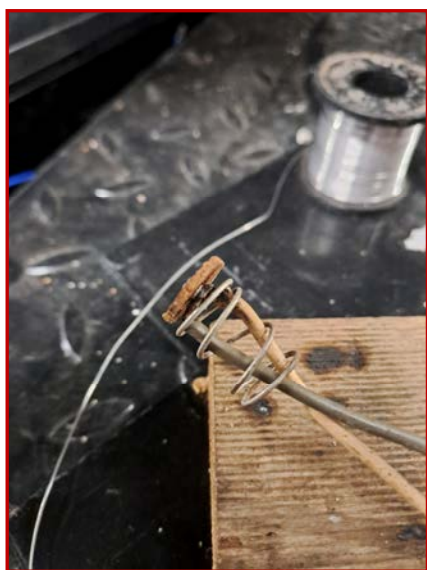
Original lamp holders needed repair.
